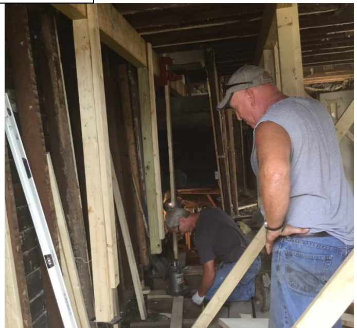
Figure 5 Right, looking north, north wall being supported by two temporary posts and beams as repairs are made to north wall. 7/19/2016. GRG photo; used with permission.
