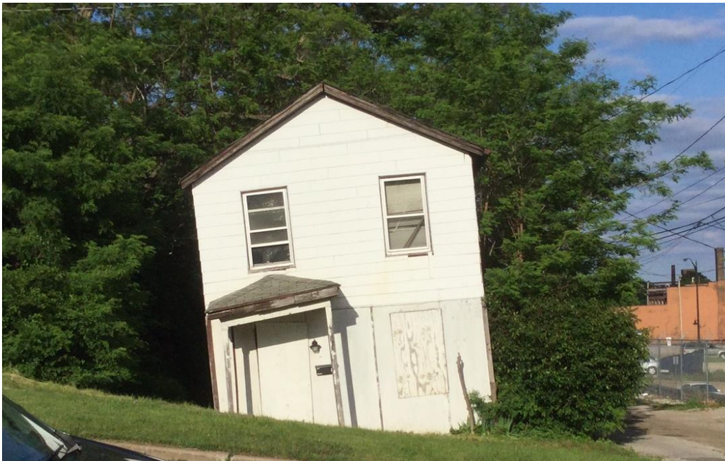
Figure 1 Looking east, the Nesbit Cottage prior to remediation showing building leaning to the north. June 1, 2015. GRG photo; used with permission.
