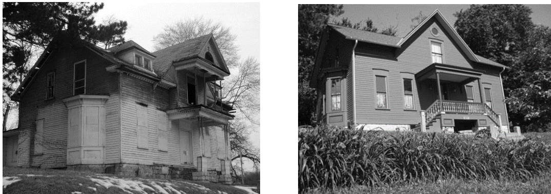
Figure 23: Before and after photos of 822 Gaines Street. A property boarded for twenty-five years and rehabbed with assistance from the HAPPEN program. [Source: Author photographs. January 31, 2005 and June 18, 2008.]
